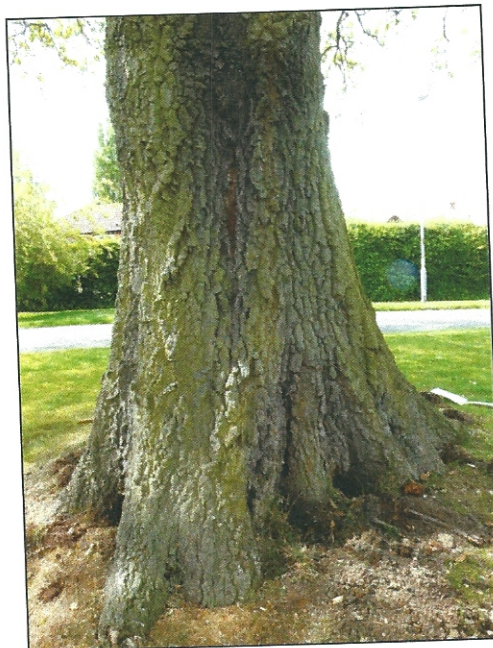
Photograph 3: Large buttress root on the southern side that has developed in response to the basal decay
